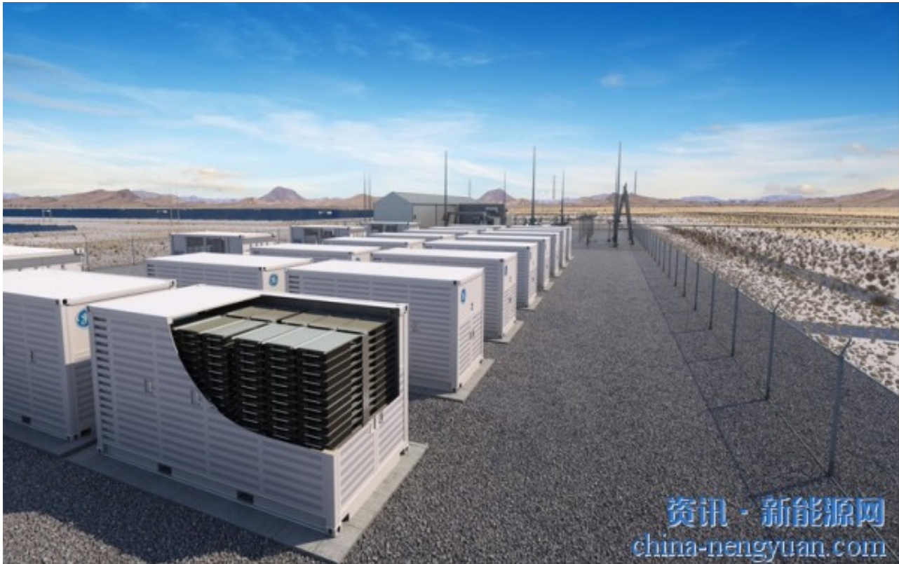
通用电气储能系统。图像：GE Renewable Energy
