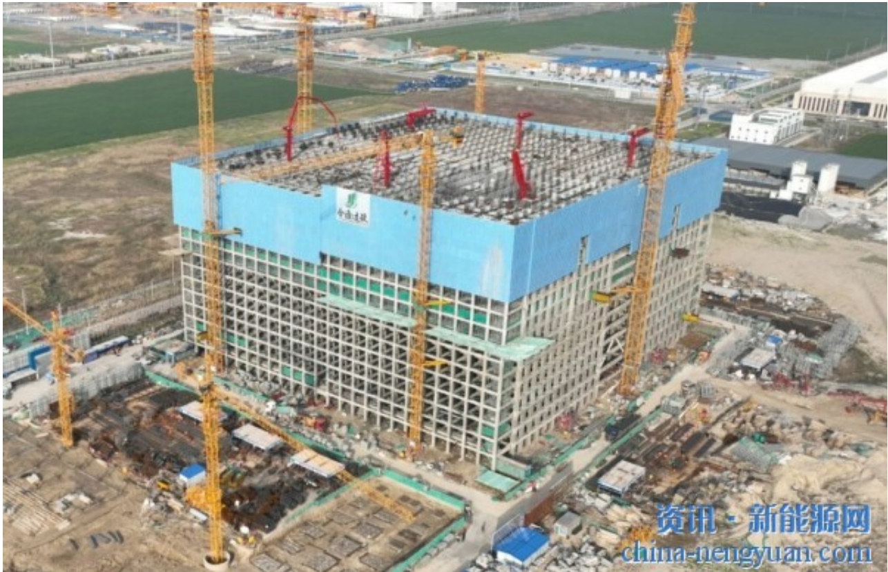
Energy Vault首个EVx系统在中国如东的施工现场。图片：Energy Vault
