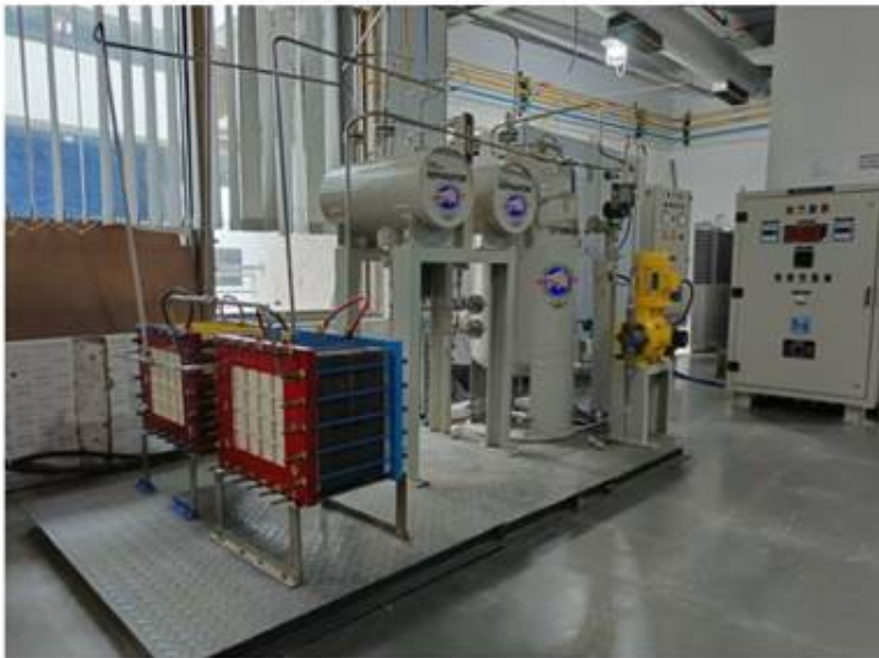
Process diagram and image of PEM based ECMR developed at ARCI with a hydrogen production capacity of 5.0 kg/day
